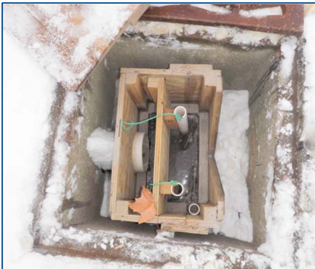
Ice and frozen sensors in catch basin weir box, Perkins Township
