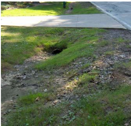
Before: Roadside swales failed to convey stormwater, causing street and yard flooding.
