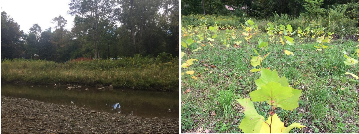
Figure 12. Post-construction conditions at the East Branch Chagrin River stream restoration project at Riverwood indicated the East Branch's access to its floodplain within the restoration reach (left) and good establishment of installed native plant species (right). Photo source: Chagrin River Watershed Partners, 2017.
