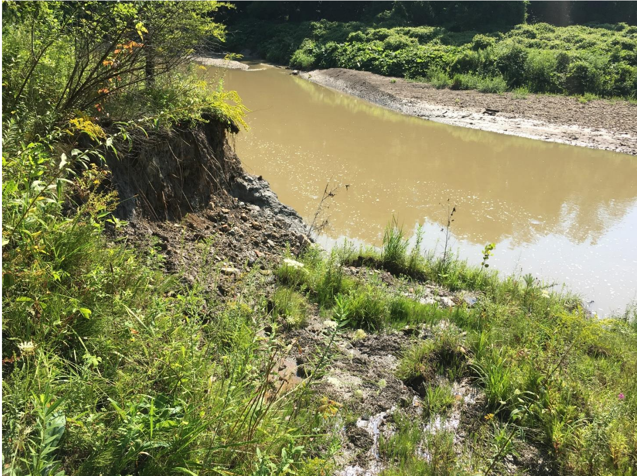
Figure 15. At one site, hardened streambanks within a streambank stabilization project reach may be contributing to erosion immediately downstream. Photo source: Chagrin River Watershed Partners, 2017.
