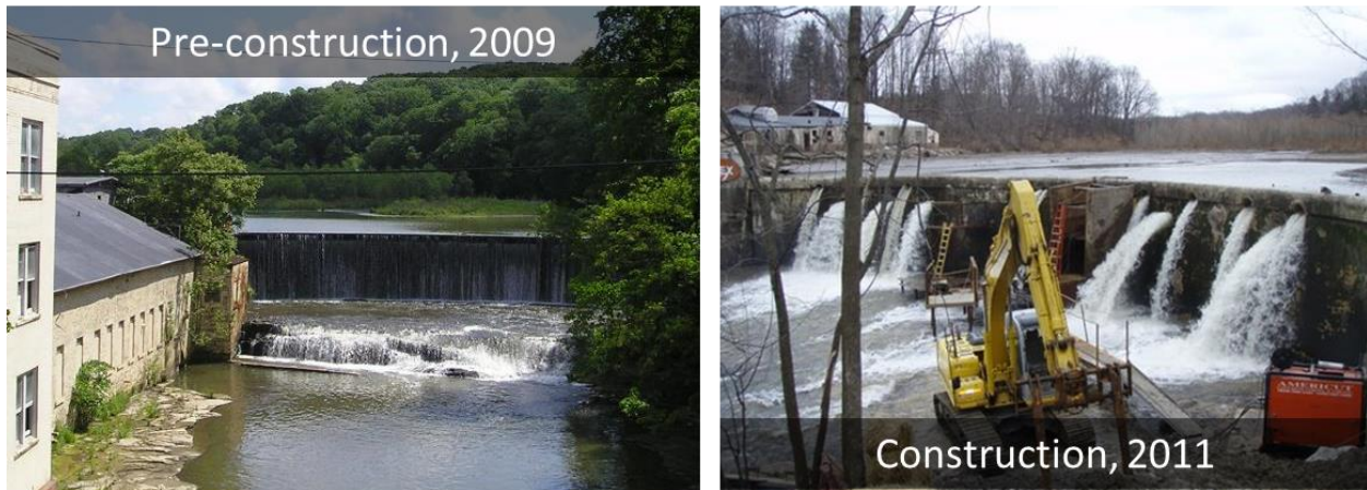
Figure 8. Pre-construction and construction conditions for the Ives of Ohio lower dam modification and stream restoration project. Photo source: Chagrin River Watershed Partners.
