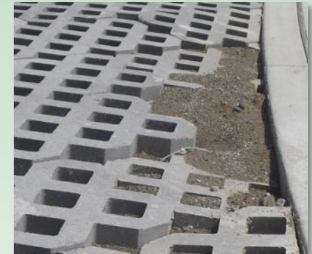
Improper Base Course
