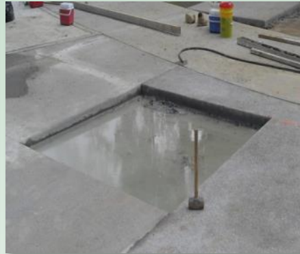
Clogged Drainage Course
