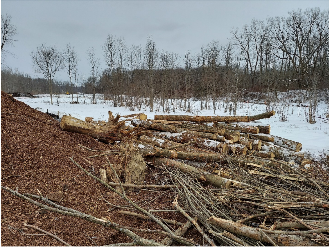
Figure 5. Woody debris materials to be used in the Beaver Creek Restoration Project during construction. Photo source: BioHabitats, February 2021.
