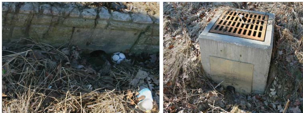
Figure 6. Unprotected Dry Basin Outlets
