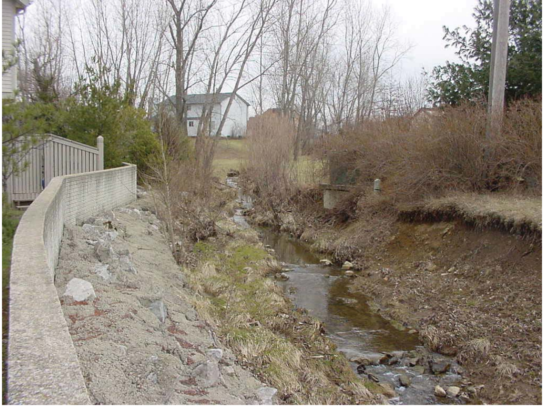
Stream instability associated with stormwater increases often brings hard and harsh solutions.
