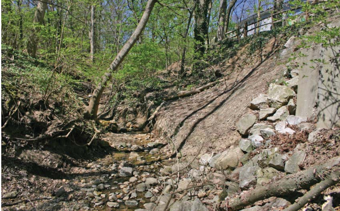
Storm water runoff to this ravine has caused over 2 feet of vertical stream erosion (incision).
