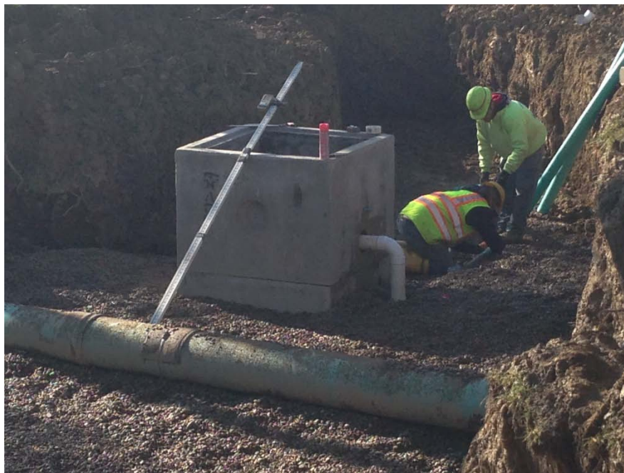
Figure 53. Internal water storage zone (IWS) installed using an upturned elbow in the underdrain at the Ursuline College bioretention cell.
