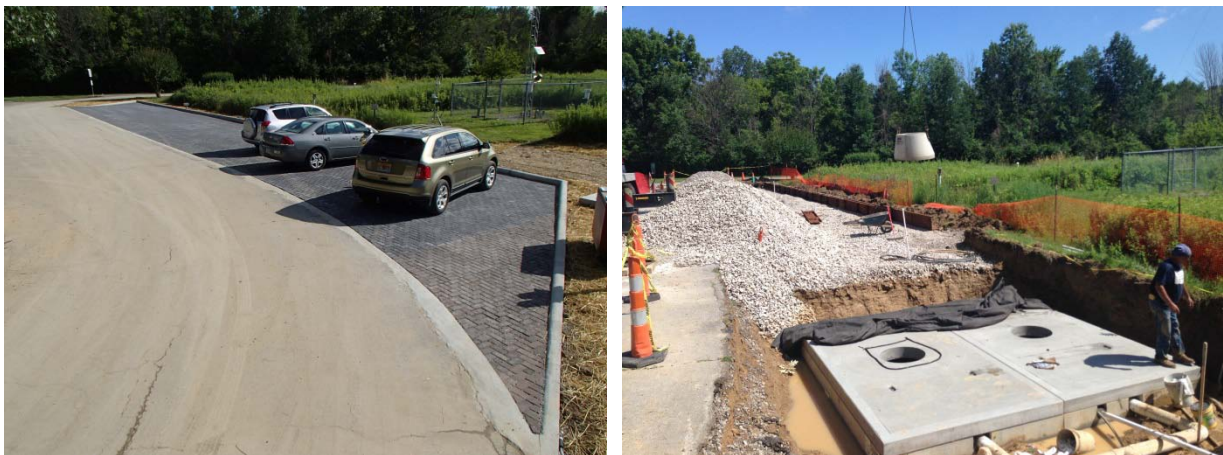
Figure 42. Permeable interlocking concrete pavers (PICP) with standard asphalt watershed (left) and underground cisterns located beneath PICP (right) at Old Woman Creek NERR.
