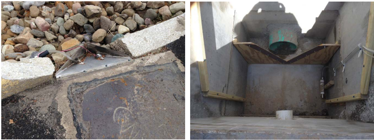
Figure 54. Inflow monitoring structure located between the parking lot and the forebay (left) and top view of weir installed in Ursuline College outlet structure (right).
