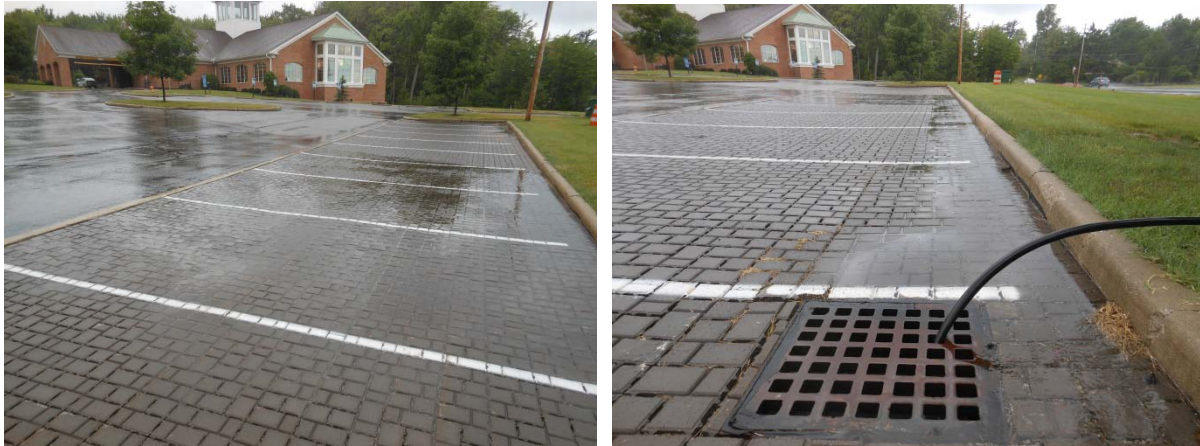
Figure 69. Runoff entering PICP at Willoughby Hills on July 17 th , 9 days after infiltration testing. Shallow concentrated flow created by parking lot island (left) and flow passing all the way to the catch basin, bypassing treatment (right).
