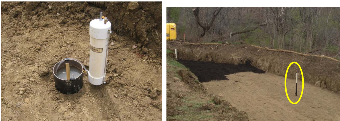
Figure 26. Single ring infiltrometer with Mariotte bottle used for pre-construction infiltration testing (left) and monitoring well used for post-construction drawdown rate measurement.
