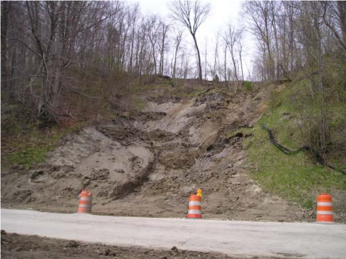
Slope failure along Chagrin River Road
