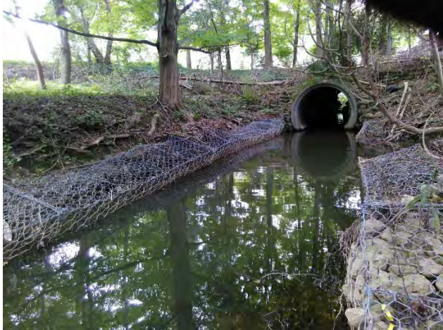
Figure 6. Gabion baskets are present at 2733 Sinton Place, Pepper Pike, Ohio.
