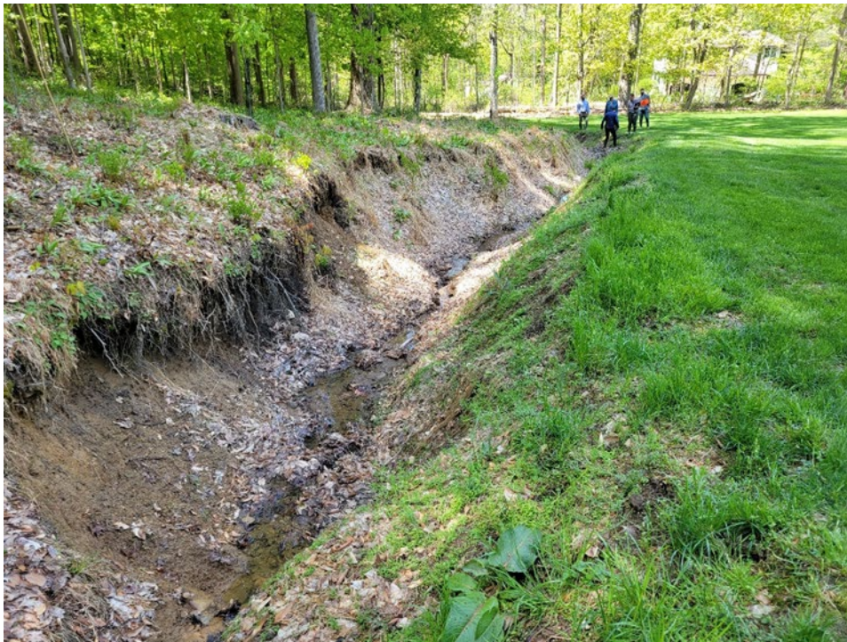
Figure 1. Eroding streambanks prior to stabilization work. Photo source: Chagrin River Watershed Partners.
