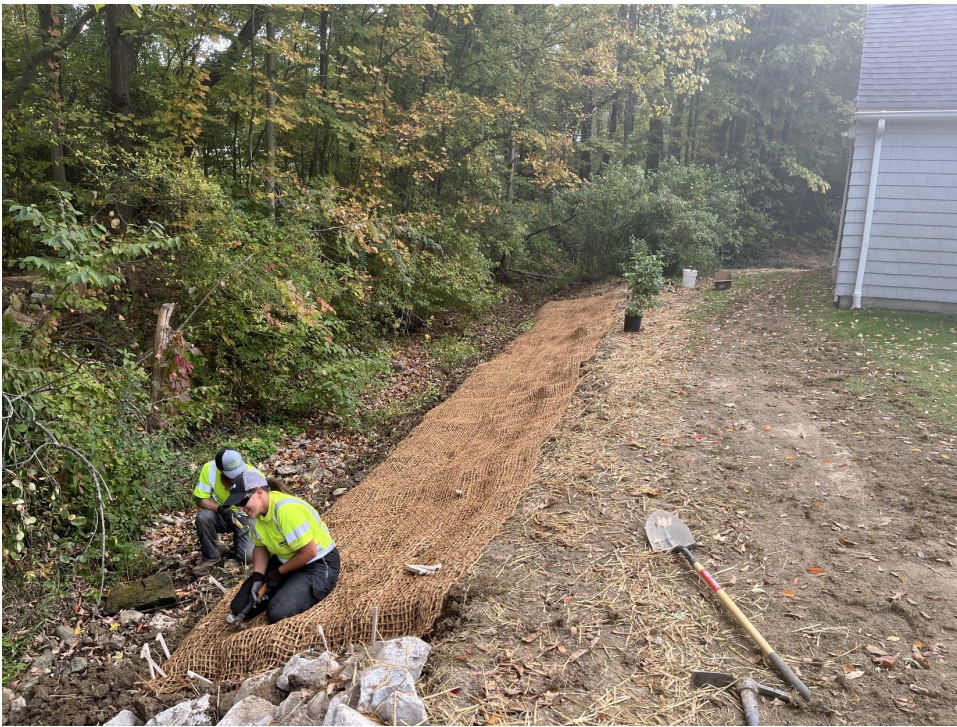
Figure 3. Streambank stabilization work is performed at a residential property by Davey Resource Group. Photo source: Davey Resource Group.
